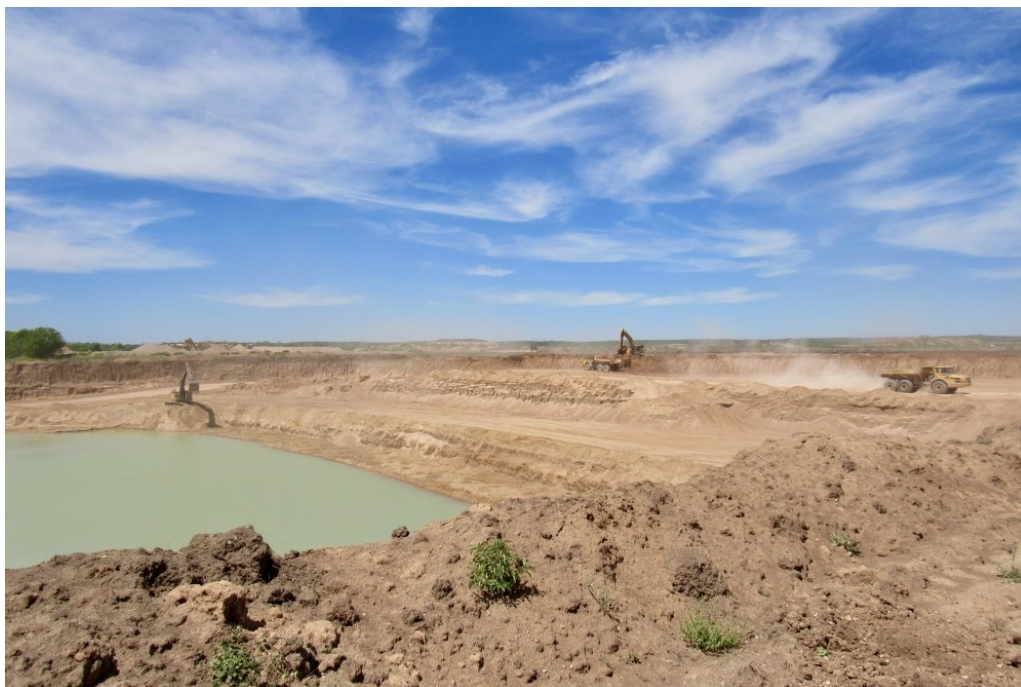
Raw material is then screened, washed and dried. Rock crushing and sorting machines used in this step are often the source of noise concerns. (Jane Turchi/Community Impact)
