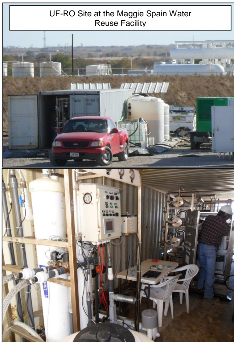
Figure 10-1: UF-RO Site at the Maggie Spain Water Reuse Facility
